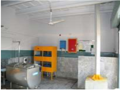
EMS System / Inverter and Alarm Bell
